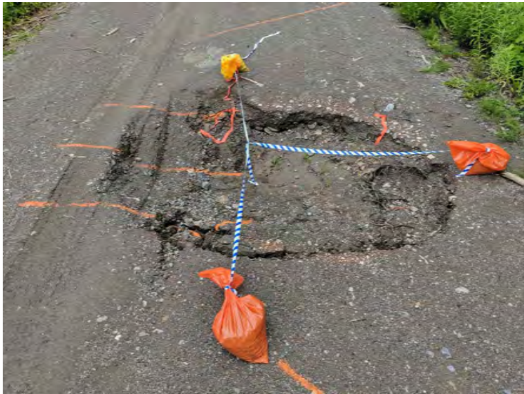
Sinkhole in Road
