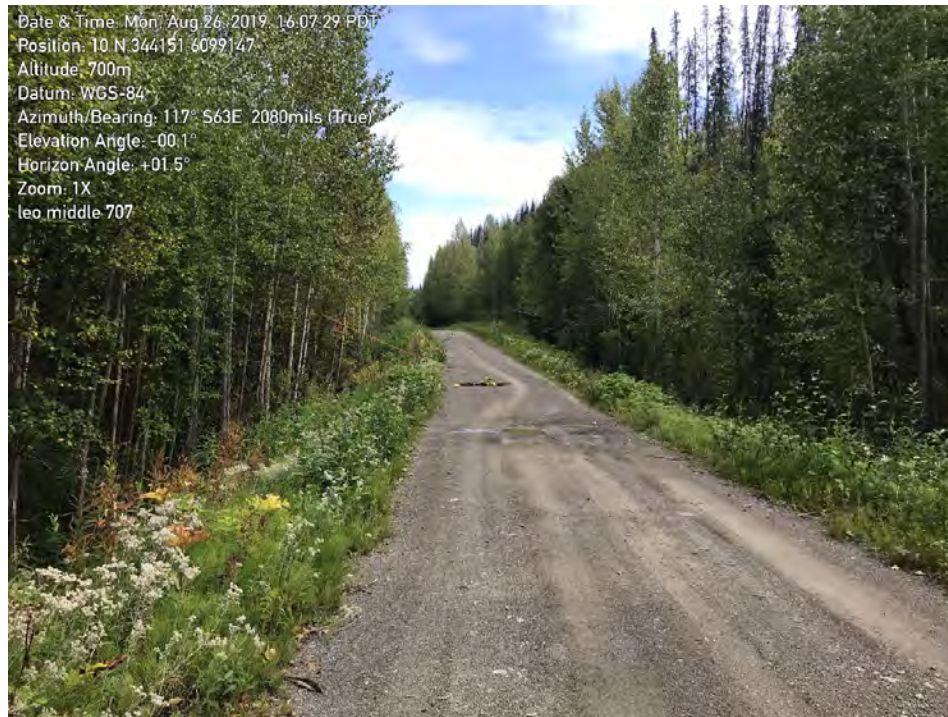
Photo 1. Road washout at Km 7, looking towards the high chain side.
